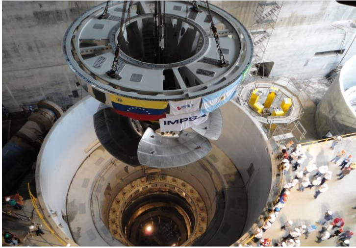
Figure 9: Lowering its first Kaplan Turbine at Manuel Piar Hydroelectric Power Plant (IMPSA)
