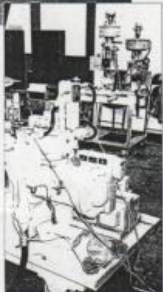
Foreground, gate shaft governor converted with parts of modular new ModuFlo distributing valve, replacing the mechanical column
